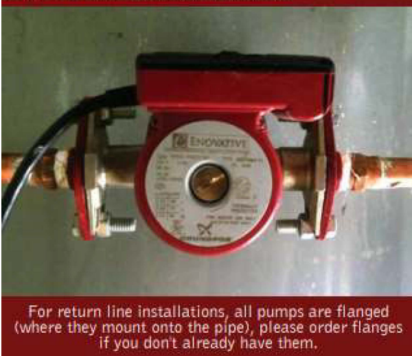
Figure 1: Pump on a return line
