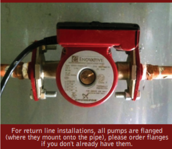
Figure 1: Pump on a return line
