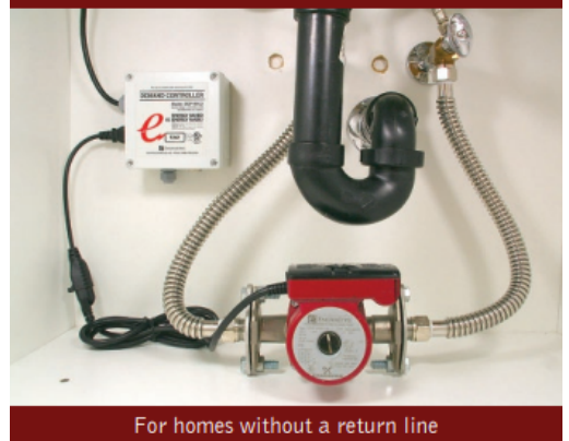
Figure 2: Pump installed under the sink with the -USK Kit
